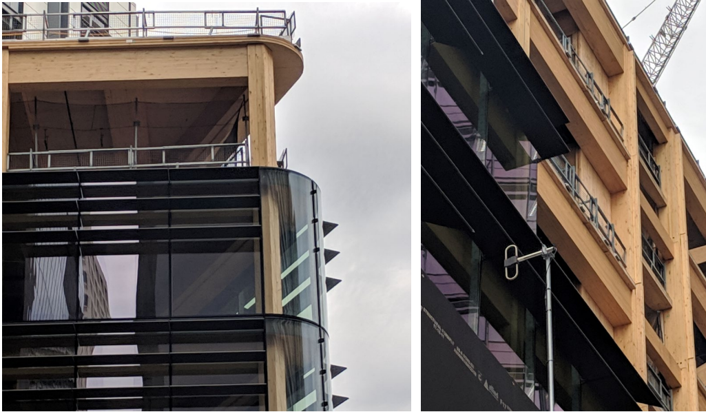
Figure 1: Example of mass timber building under construction using CLT slab construction (Photo: Carl Pettersson)
