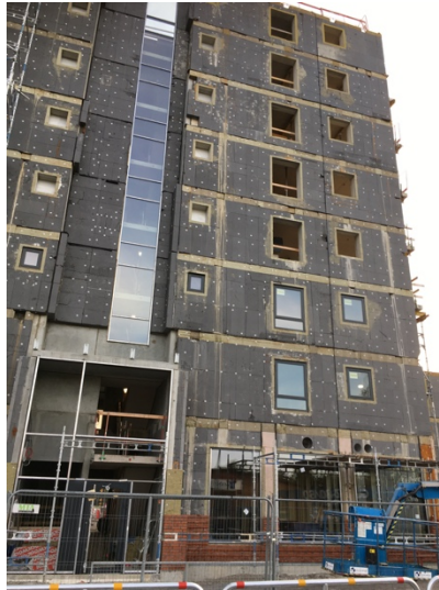
Figure 33 Example of the introduction of fire stopper in a combustible insulation of a façade and where no vertical fire stoppers are placed (picture Patrick van Hees)
