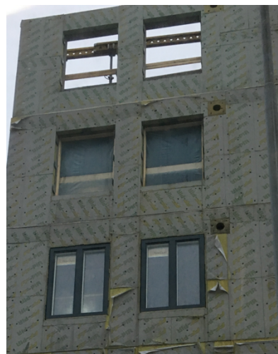
Figure 34 Example of need for detailed finished of possible protection layers of the insulation material (picture Patrick van Hees)
