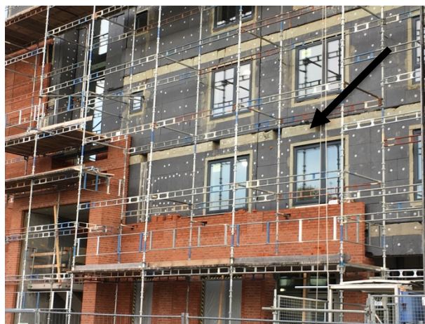
Figure 32 Example of the introduction of fire stopper in a combustible insulation of a façade system where the external layer is non-combustible (picture Patrick van Hees)
