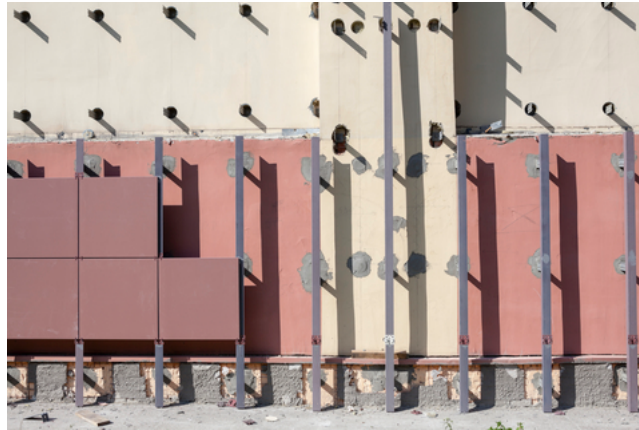
Figure 19 Example of a rainscreen cladding under construction (picture courtesy ID 44710574 © Antikainen | Dreamstime.com)
