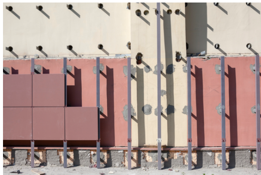
Figure 2 Example of a complex rainscreen façade systems (picture courtesy ID 44710574 © Antikainen | Dreamstime.com)
