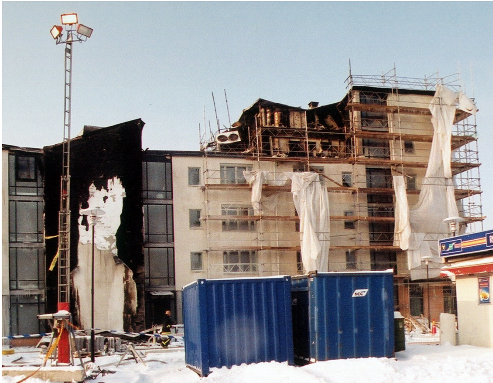
Figure 31 Example of fire spread from the attics into a rendered façade system (picture courtesy RISE)
