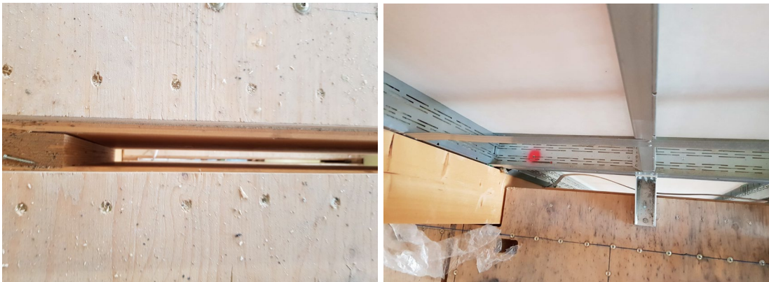
Figure 8: Example of gaps in floor slab (left) and curtain wall system (right) in a timber building during construction. (Photo Carl Pettersson)
