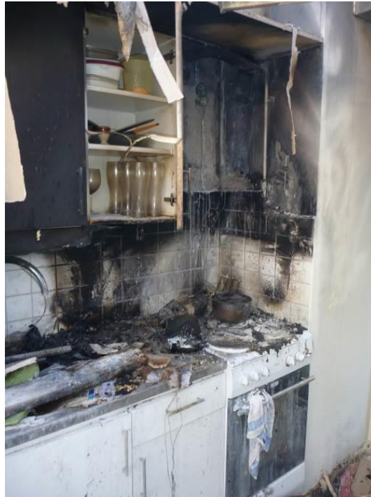
Figure 4 - Fire damage after extinguishment of the fire in the ignited compartment 2
